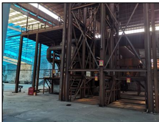
冰铜车间内富氧侧吹还原炉
